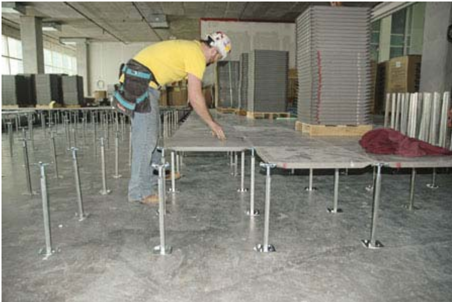
Installation of the UFAD system at Great River Energy. The UFAD provides 30% additional fresh air delivery to occupants and 50% energy savings. Photo: Courtesy of Tate Access Flooring
